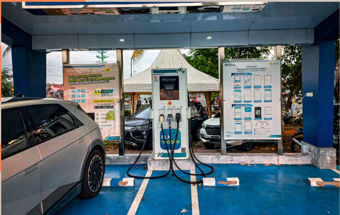
EV charging station in Central Java, Indonesia.
